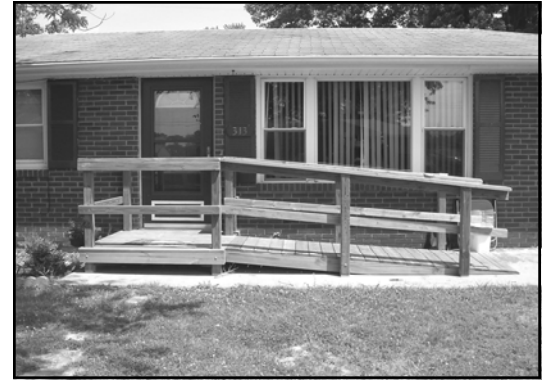
This ramp was built in front of Mr. Baatz's daughters' home in Hanover so he could remain independent.
